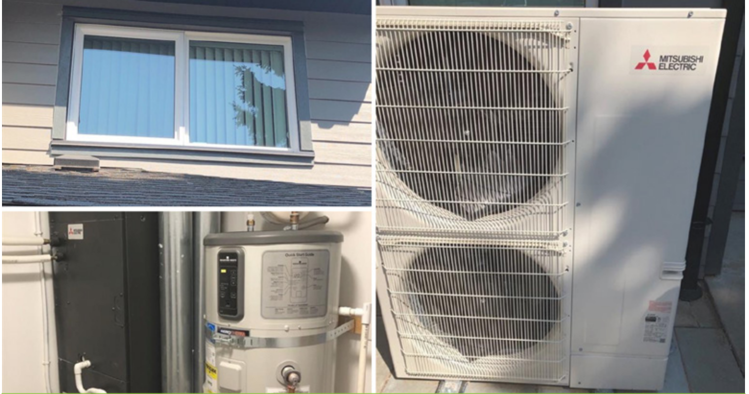
A Deep Energy Retrofit project at Kinsmen Ravine which included central heat pump outdoor units, domestic hot water heat pumps, and windows upgrade.
