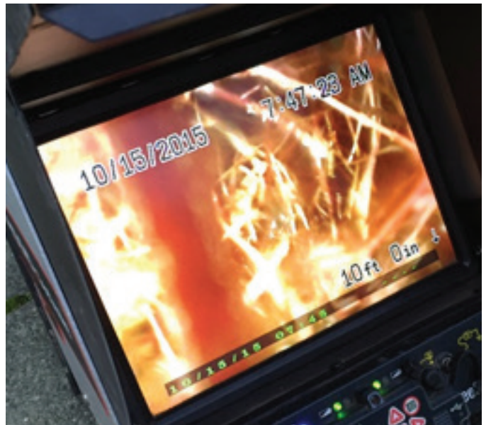
Figure 10.3 Camera view of drain pipe infilled with roots.
