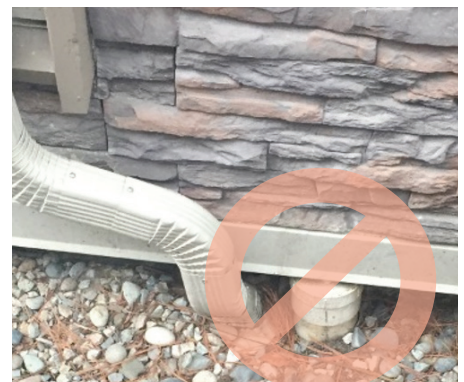
Figure 9.2 Cleanout blocked by the flashing at the base of the building's wall.
