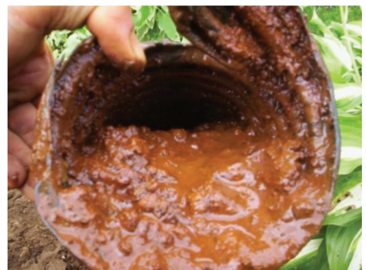
Figure 9.3 Iron ochre in a drainage pipe.
