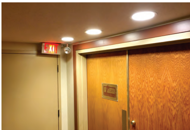
LED pot lights and old Exit signs
