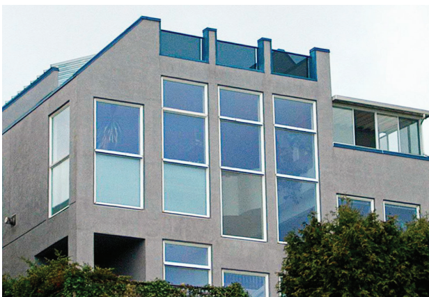
These windows are exposed to wind-driven rain. Water resistant products and installation methods must be used.
