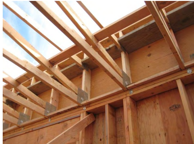
A wood-frame multi-unit residential building (MURB) under construction—how much insulation is needed in the wall and roof assemblies for energy code compliance, or to meet the requirements of a high-performance building?
