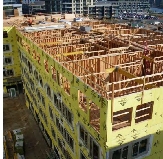
Construction of a 6-storey MURB with non-combustible gypsum sheathing. Framing factors at lower floors are higher than at upper floors in order to accommodate structural loads. The effective R-value of these walls will be affected by this wood-framing factor and the chosen insulation strategy.
