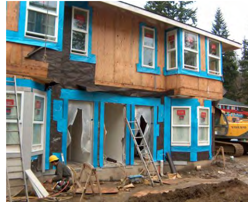
Excessive and improper use of vapour-impermeable, self-adhered membrane (blue) around windows and other penetrations of a wood-frame building in Climate Zone 5.
