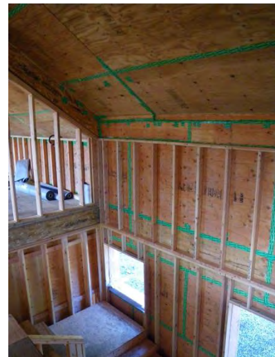
A rigid, interior, air-barrier approach using taped plywood sheathing at the inside of the wall assembly is common in Europe and many Passivhaus designs with highly insulated wood-frame walls (pre-fabricated and site built).
