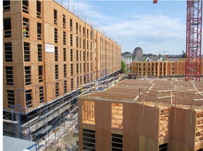
A mixed use multi-unit wood-frame building development under construction in Marine Climate Zone 4 in Seattle, Washington.
