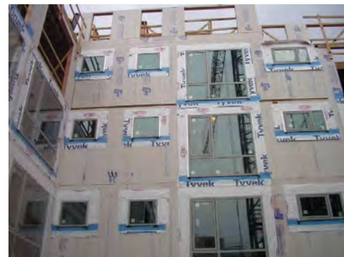
Minimal and proper use of impermeable, self-adhered membrane (blue) at window sills, with vapour-permeable membrane used at the jambs and head of the windows of a wood-frame MURB in Climate Zone 4. Window detailing is covered in further detail in Chapter 6, complete with build-slides that show sequencing of this detail.
