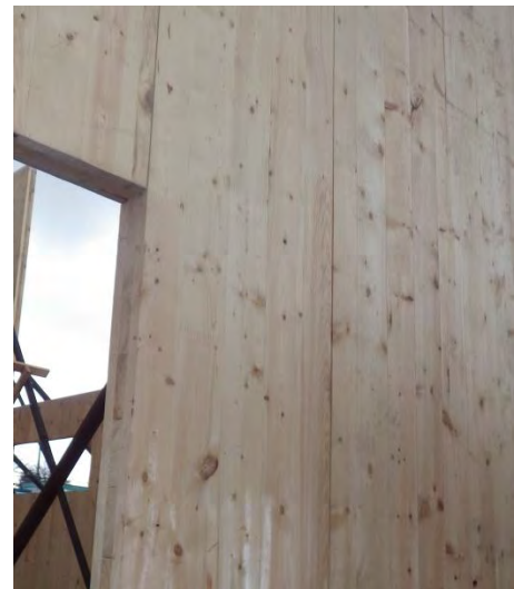
Shrinkage gaps between the wood pieces and panels in service make CLT panels generally difficult to make air tight, therefore a separate air barrier membrane is recommended.
