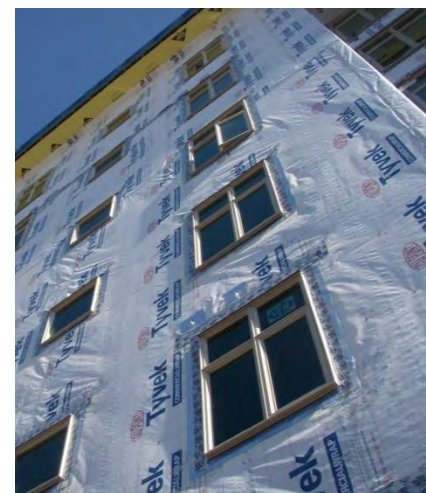
When properly detailed and supported during construction and in-service, the exterior, sealed sheathing membrane, air-barrier approach can be a successful strategy for air-flow control in a MURB.
