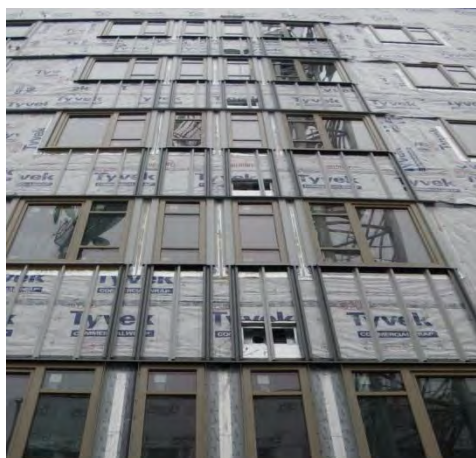
There is very little test data available to allow for a more analytical or even empirical approach to determining the structural adequacy of sheet-membrane barrier systems. Precautionary measures could include tightly spaced strapping to secure the membrane, and selection of more robust membranes (i.e., in terms of strength and tear resistance). The use of self-adhered and liquid-applied membranes basically makes the sheathing and membrane an integral, rigid, air-barrier material.
