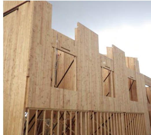
Large CLT wall panels make up most of the structure of the building and provide a substrate for the water resistive barrier and exterior insulation.
