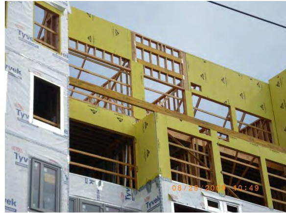
Five-storey multi-unit residential building under construction. The selection of thermally efficient assemblies is summarized in this chapter, but the details of integrating these assemblies with penetrations, windows, doors, balconies, etc. is covered in Chapter 5.
