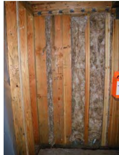
Fibreglass insulation placed between wood framing in a 5-storey MURB under construction. The effective R-value of the wall assembly is much less than the R-20 nominal batt insulation due to thermal bridging of framing, particularly when heavy timber elements are used at lower floors.
