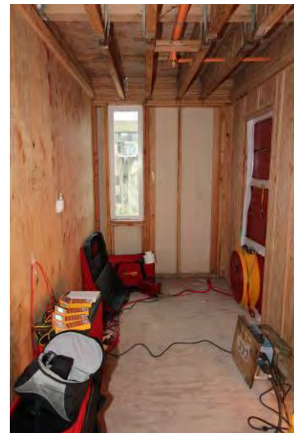
Air-leakage testing of a single suite in a wood-frame MURB. Testing is often performed as part of building commissioning to measure the enclosure airtightness as well as the compartmentalization of the individual suites prior to whole building airtightness testing.
