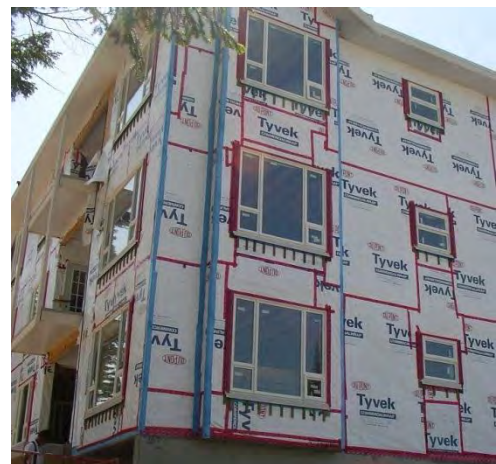
Notice the use of tapes to seal the sheathing membrane for this 4-storey MURB. Rigidity and support of the membrane will be added in the form of vertical wood strapping to create the cavity for the rainscreen wall assembly.
