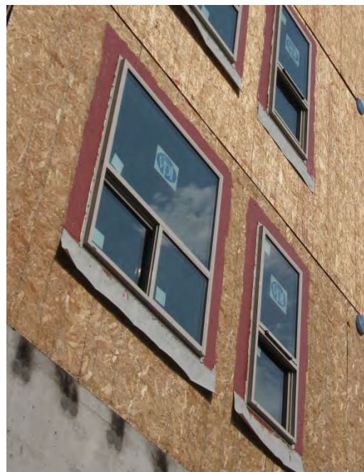
Liquid membrane used in the window rough opening to simplify sequencing and detailing.
