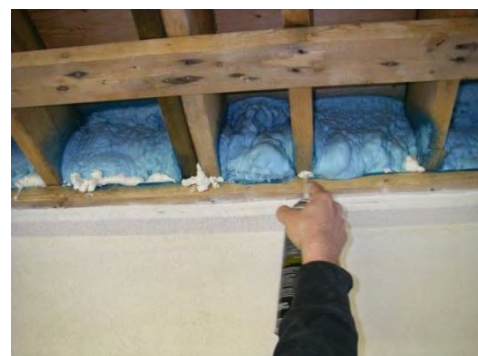
Polyurethane spray foam is used as a transition air-barrier material to seal and insulate the space between roof and floor framing. The use of spray foam to fill small to large gaps in conjunction with other air-barrier strategies is common.
