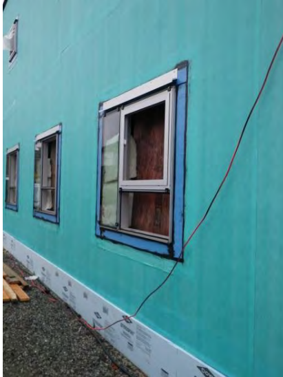
At this 3-storey wood-frame recreational building, self-adhered vapour-permeable membrane is applied directly over plywood to form the air-barrier system. Self-adhered membranes may improve detailing and provide a more rigid and durable air-barrier system than sheet applied and taped membranes.
