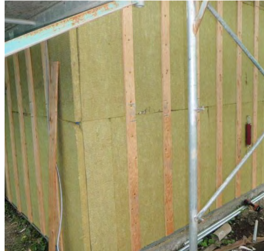
Split-insulation wall assembly consisting of rigid mineral fibre on the exterior of the wood sheathing and sheathing membrane. Cladding will be attached to the vertical strapping on the exterior of the insulation, which has been fastened back into the structure using longer screws.
