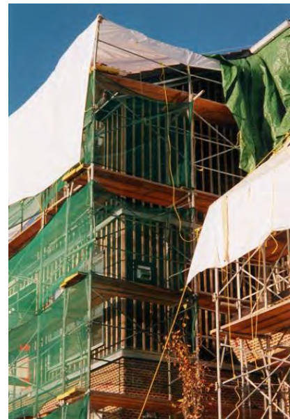
Wood-frame MURB undergoing a building enclosure rehabilitation to address moisture ingress damage. Thermal improvements to the building enclosure can easily be made when this type of work is already being performed for incrementally much lower costs than doing the work solely for an energy upgrade.
