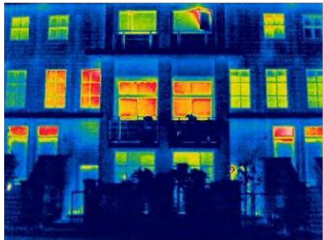
Infrared image of typically insulated, wood-frame walls (effective R-value 16.9). The windows (R-2.85), which are minimally code compliant in this jurisdiction, occupy a large percentage of the building enclosure and comprise the largest component of conductive heat loss. Standard window-to-wall ratios are, on average, between 15 and 20% for single-family houses but are much higher for MURBs. Window-to-wall ratios in the range of 30 to 50% are common for wood-frame MURBs.
