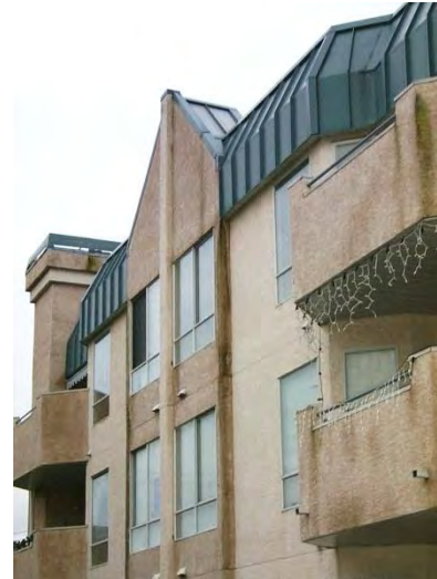
The lack of appropriate protection of the face seal stucco walls and poor interface detailing have resulted in the deterioration of many wood-frame building enclosures in wet climate zones.
