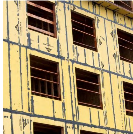
The exterior, sealed-sheathing, air-barrier approach is a rigid and durable strategy for a wood-frame MURB that meets the five requirements for an air-barrier system.
