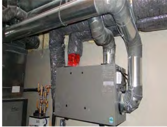
Fig. 4.5 HRV installation with trunk and branch ducting. Insulated ducts are to/from outside.
