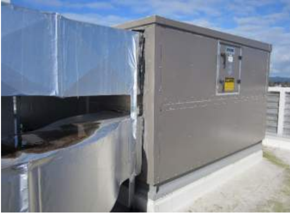
Fig. 4.4 Custom centralized outdoor HRV for an 11-storey MURB. The unit supplies ~6000 cfm to 90 units.
