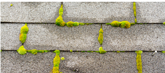
An accumulation of moss will tend to hold moisture on the roof, preventing proper drainage and accelerating the deterioration of roofing components.
