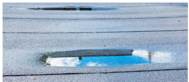
A large blister on this two-ply, low-slope roof has caused the membrane to move at the seam. The membrane has split under this stress and the blister is now full of water.
