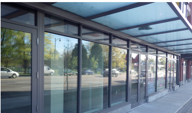
Figure 6 – Example of storefront glazing on the commercial first floor of a mixed-use building
