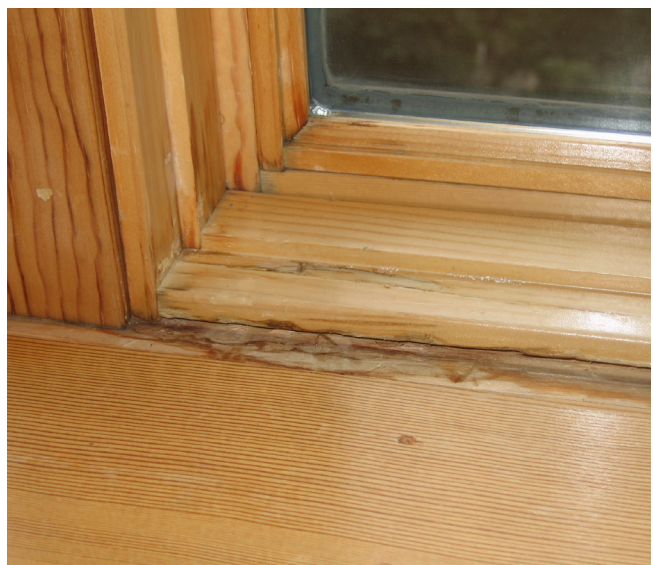
Figure 8 – Staining on interior surface of existing wood windows
