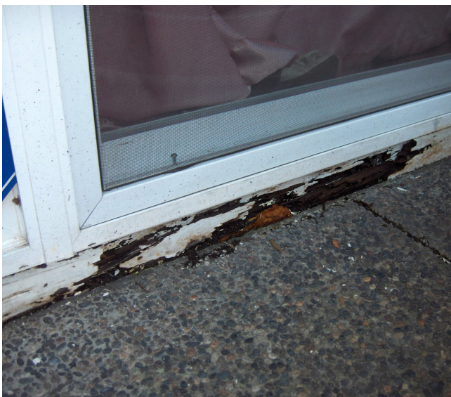
Figure 7 – Decay of exterior wood trim board under door
