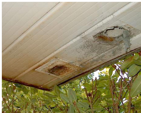
The build-up of debris or dirt on the underside of the balcony limited the air flow through the vent, resulting in damage.
