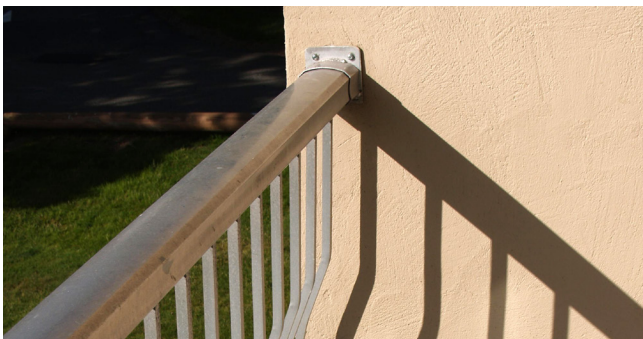
Guardrail connection to the wall can be a vulnerable point of water ingress.
