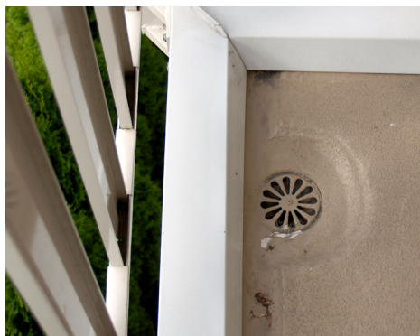
Maintain drains free of obstructions, dirt or debris to ensure they are free flowing and to prevent water ponding.
