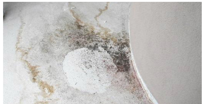
Staining on this deck membrane indicates ponding. Holes or punctures must be repaired as soon as possible to avoid water entering the structure when it rains.
