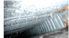
Condensation at the duct outlet.
