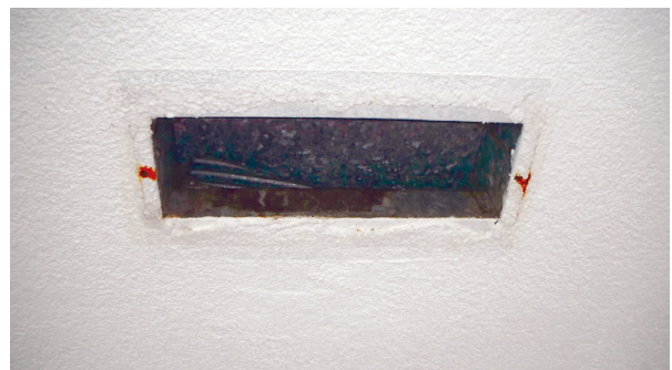
Indications of condensation build up.
