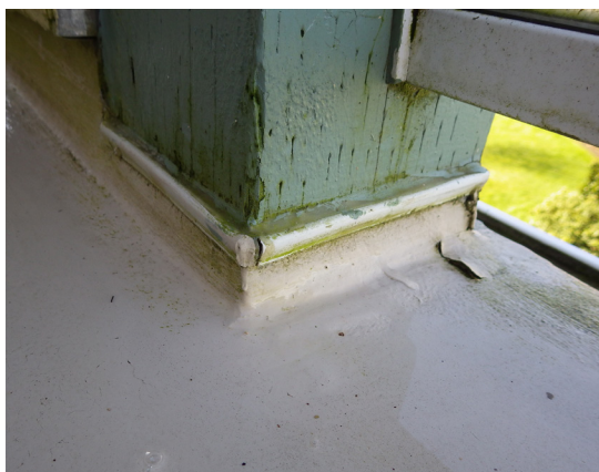
Figure 4 - Failure of the balcony membrane
