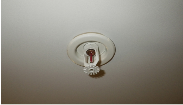
Example of a ceiling mounted sprinkler head in a wet fire suppression system
