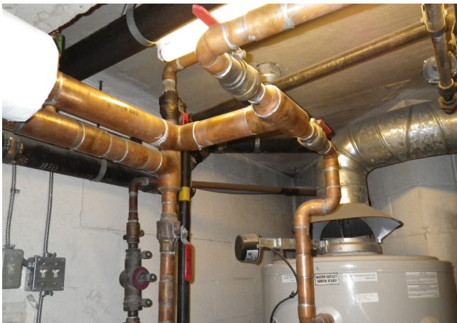
Example of un-insulated copper piping
