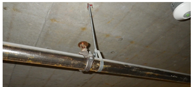
Example of a pipe mounted sprinkler head in a dry fire suppression system in the garage of a multi-unit residential building
