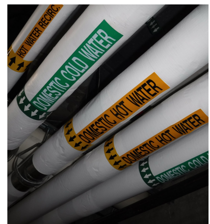
Example of domestic cold water and hot water piping wrapped in insulation
