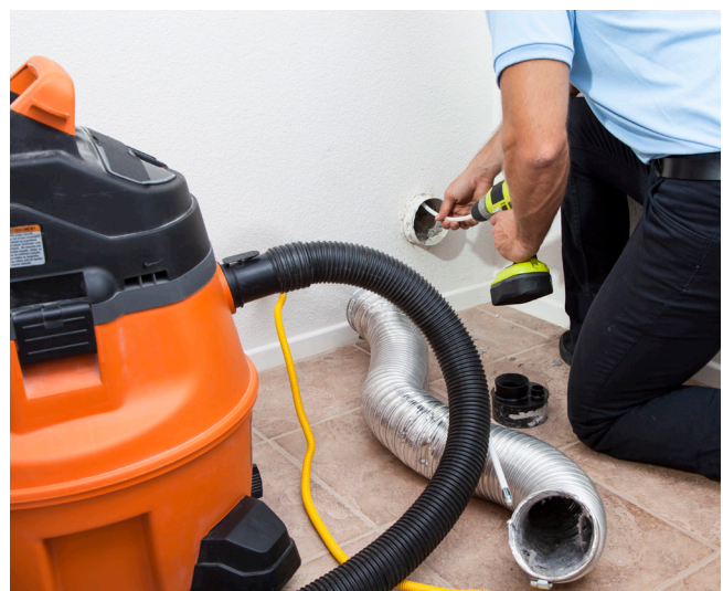
Cleaning and maintaining dryer exhaust vents
