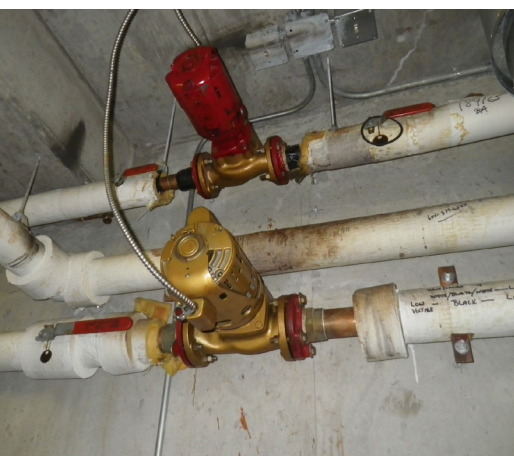
Pipe-mounted domestic hot water circulation pumps recirculating hot water from system
