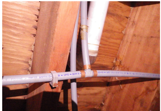
Example of polybutylene piping used for in-suite water distribution
