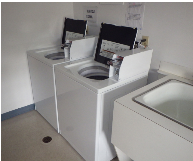
Example of a communal laundry room with a built-in drain in case of washing machine back-up, overflow or leaks
