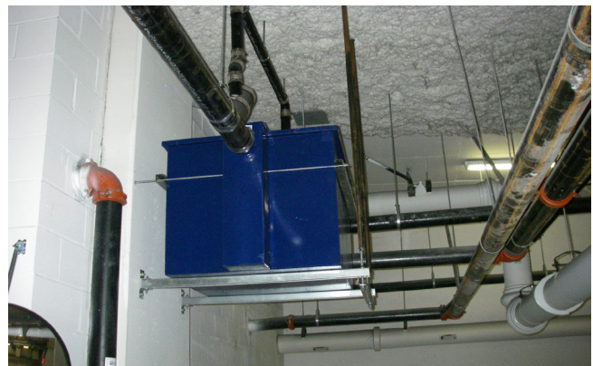
Example of a multichambered flow through grease trap suspended from the structure above
