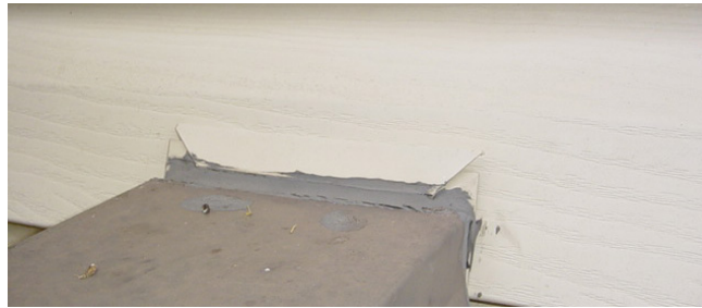
The sealant at the guardwall connection to the wall has begun to fail; a regular inspection and maintenance plan will detect this type of failure before it converts into a costly repair item.
