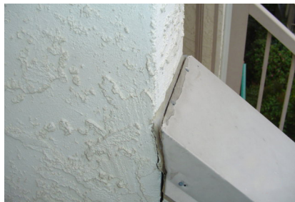
Lack of adhesion between sealant, flashing and stucco will allow water ingress at this building detail (balcony connection).
