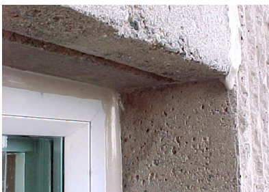
Sealants are used at many different locations in the building envelope. They are important building components and must be adequately inspected and maintained.
