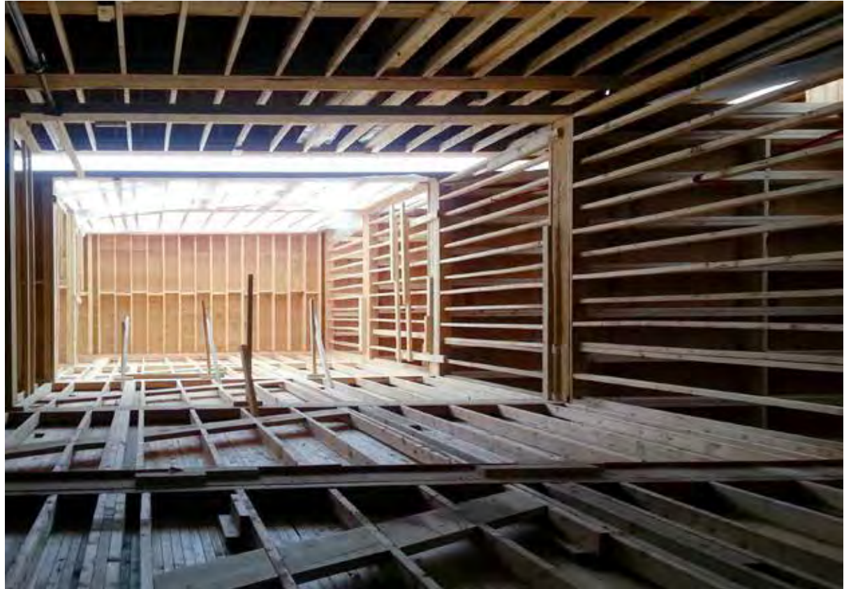
FIGURE 5.3 – HILLCREST VILLAGE: AS IS TYPICAL IN MID-RISE CONSTRUCTION, STAIR WELLS ARE CONSTRUCTED WITH LIGHT WOOD-FRAME ELEMENTS
