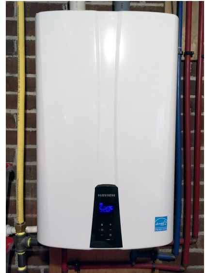
An on-demand domestic hot water heater in a home
