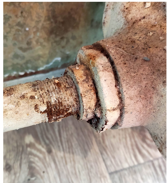
Example of a corroded pipe joint
