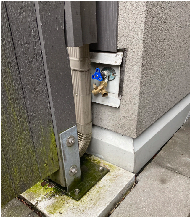
Exterior faucets should be checked annually for leaks and signs of deterioration
