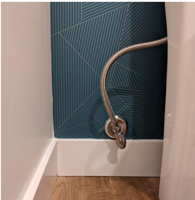
Braided metal hoses such as these are far more resistant to leaks compared to standard rubber hoses. Inspect braided metal hoses for breaks in the stainless steel protection
