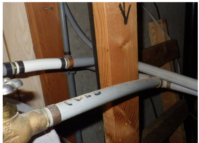
Polybutylene piping for domestic hot water in a residential home
