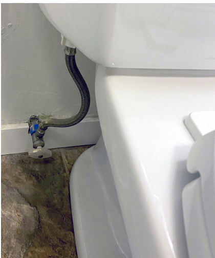
Water shut off valve for a toilet connection, which may be shut off if needed
