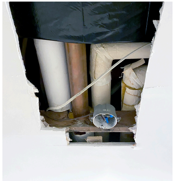
Water circulation pipes in mid-repair after a slow leak was observed by a wet stain in the drywall
