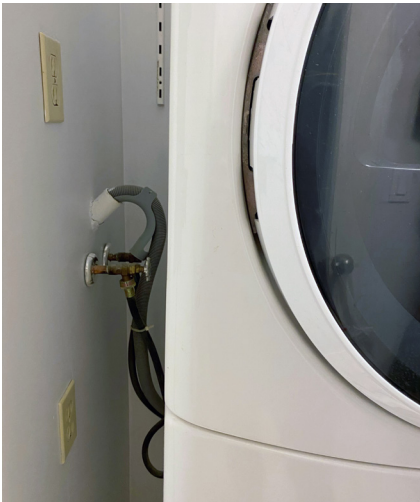
Water faucet for washing machine connection, which may be shut off if needed
