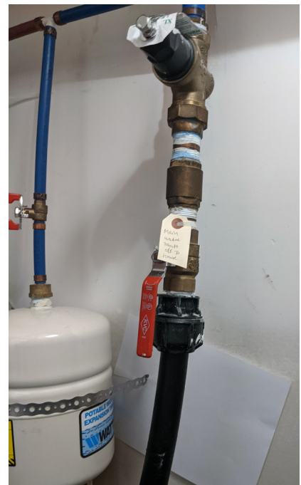
A main water shut off valve in a single-family dwelling
