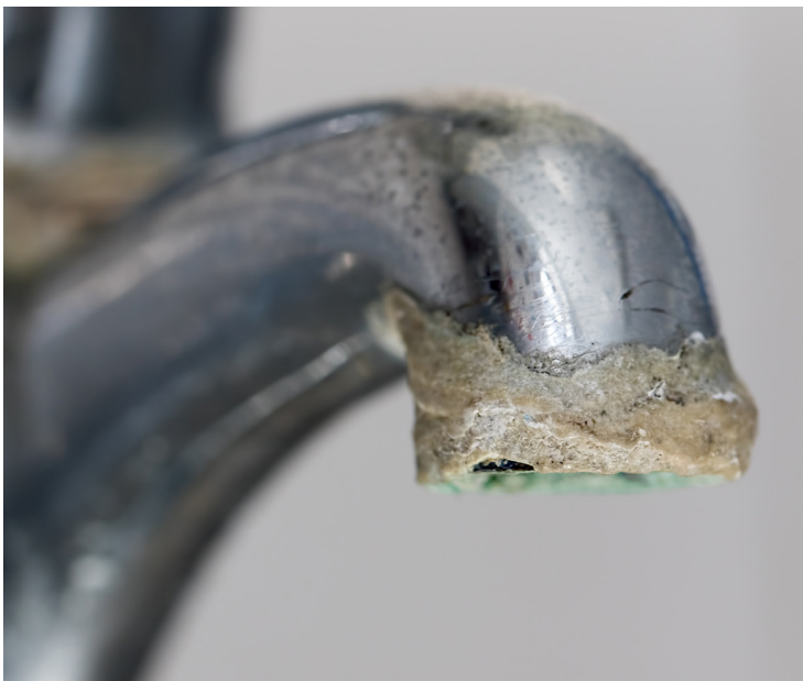
Mineral buildup on a sink tap that can cause damage or clogging
