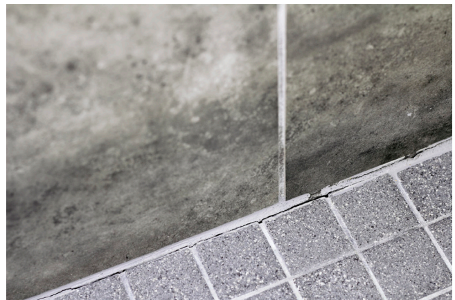
Example of sealant around a shower that is in need of replacement
