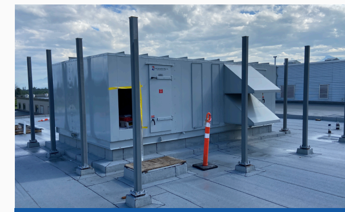
Figure 7. Figure showing anchor penetrations into the roof.
