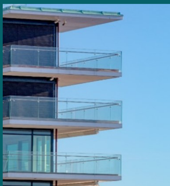
Figure 5. Cantilevered external balconies get a lot of attention as thermal bridges but less obvious thermal bridging at roof decks require equal consideration.
